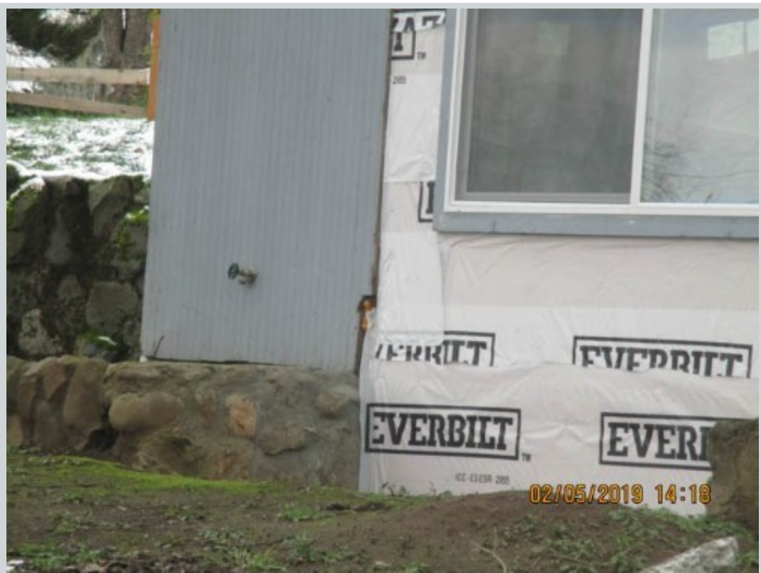
Subject 4210 Ne 39th St Comment "missing siding"
