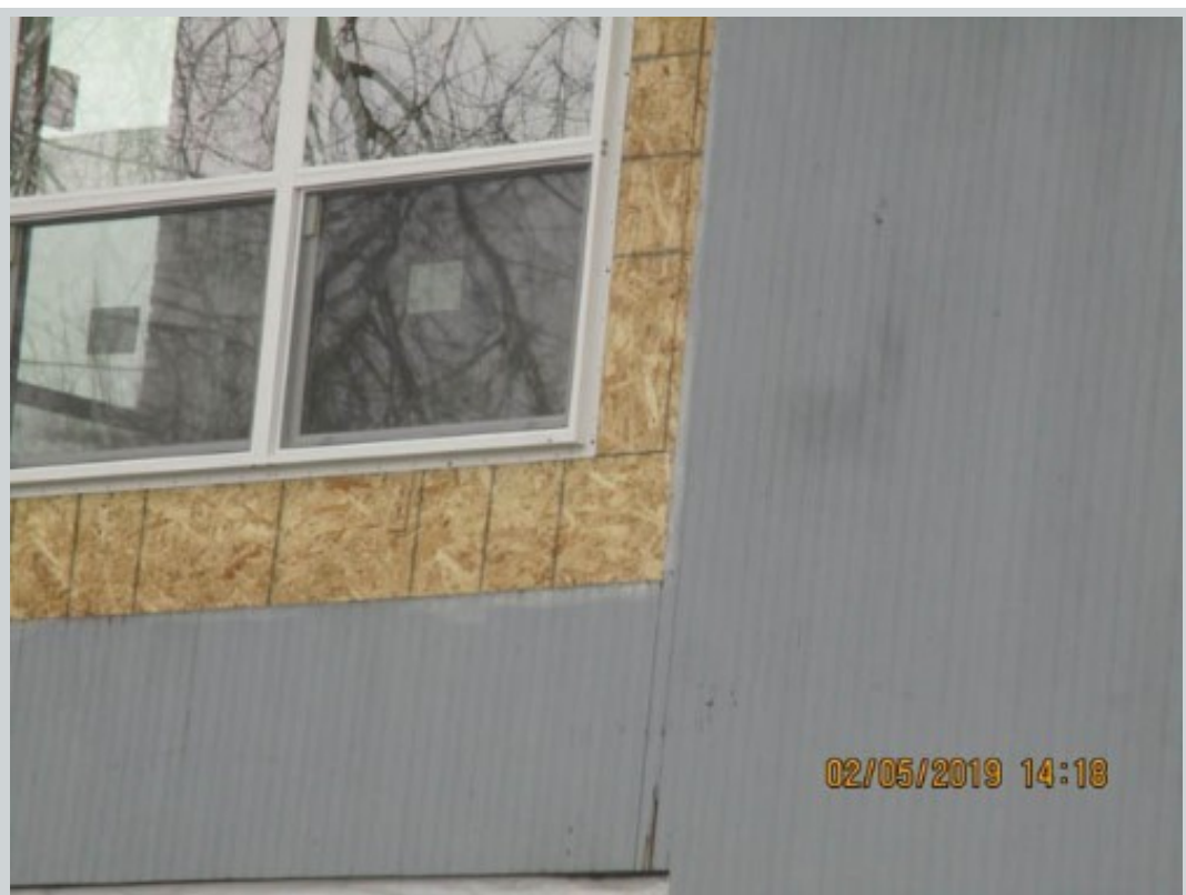
Subject 4210 Ne 39th St Comment "missing siding"
