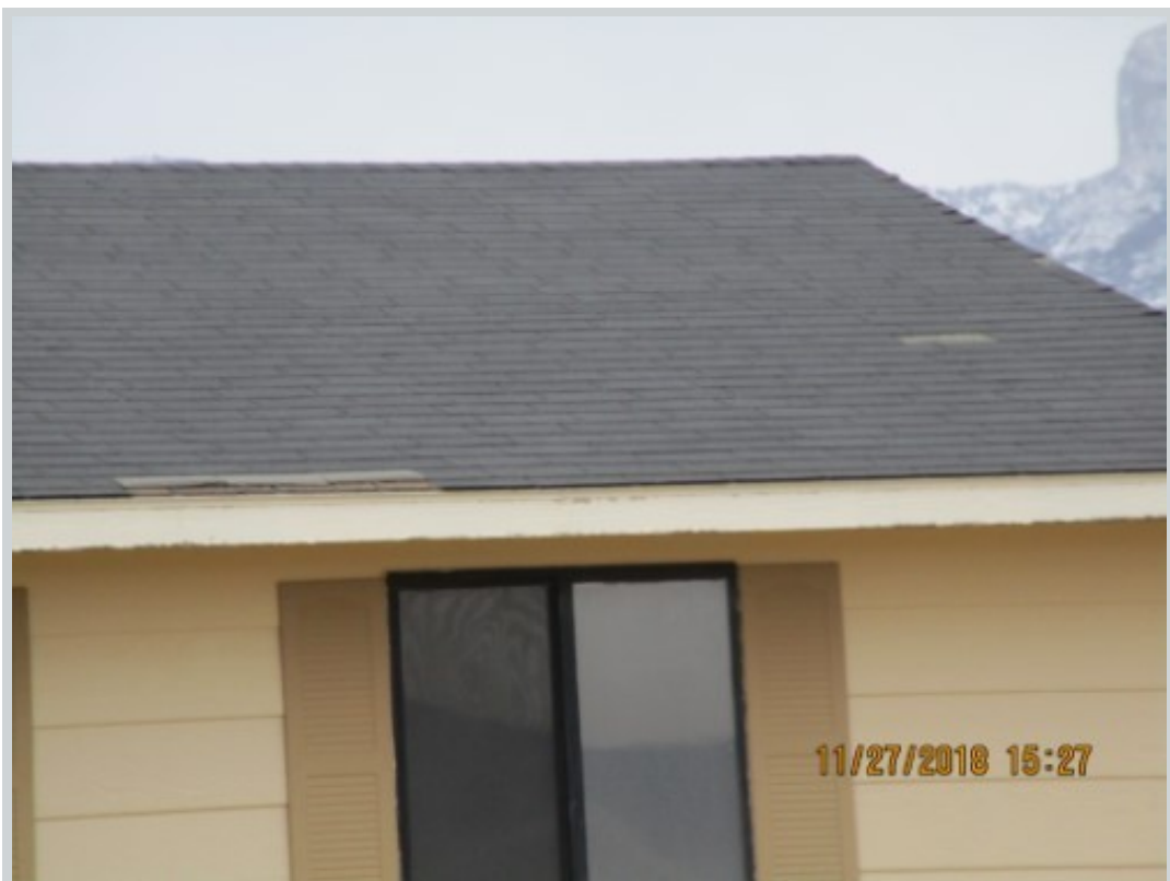
Subject 802 Royal Oak Dr View Other Comment "roof condition"
