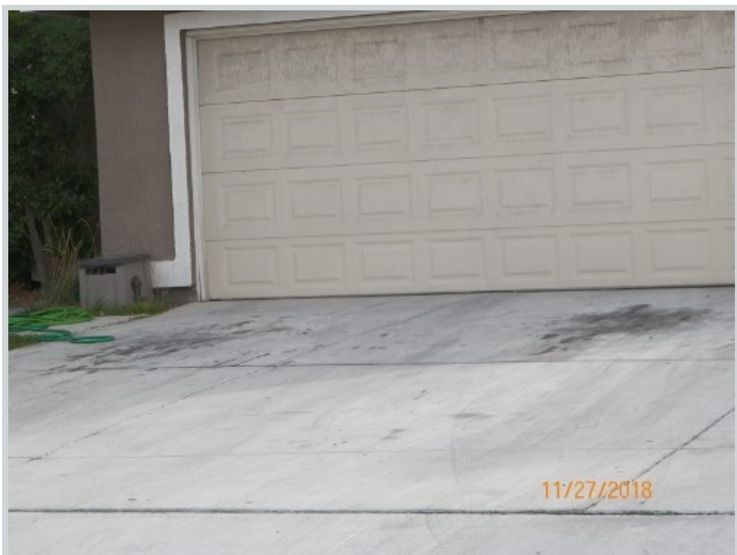
Subject 13025 San Carlos Ct View Other Comment "stained driveway"
