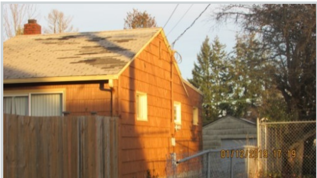
Subject 1515 S Trafton St View Other Comment "roof damage and paint"
