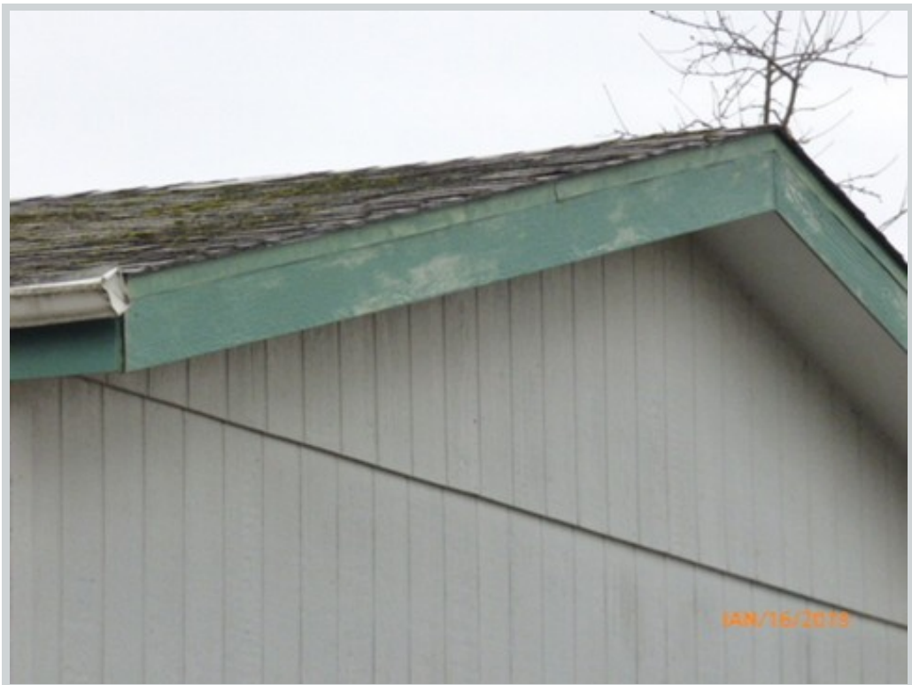
Subject 1988 Michigan City Ln Nw View Other Comment "Bare wood on trim needs painted."
