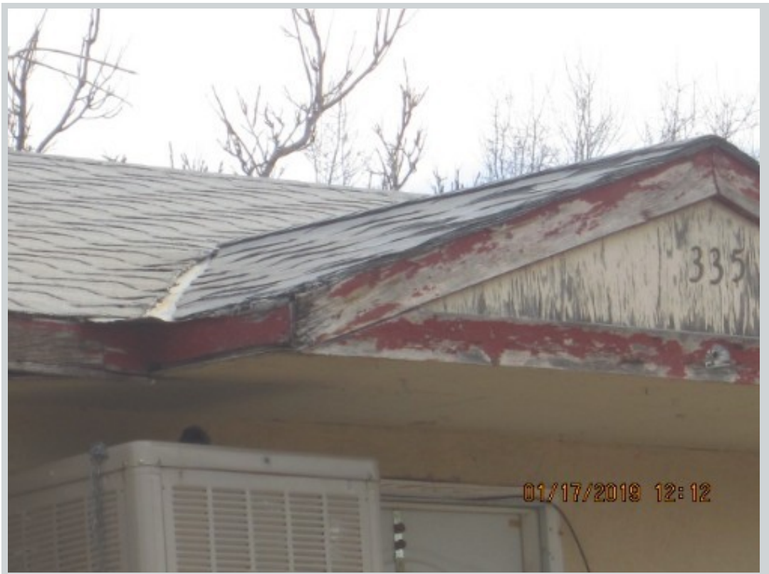
Subject 335 Lucille St Comment "peeling paint"
