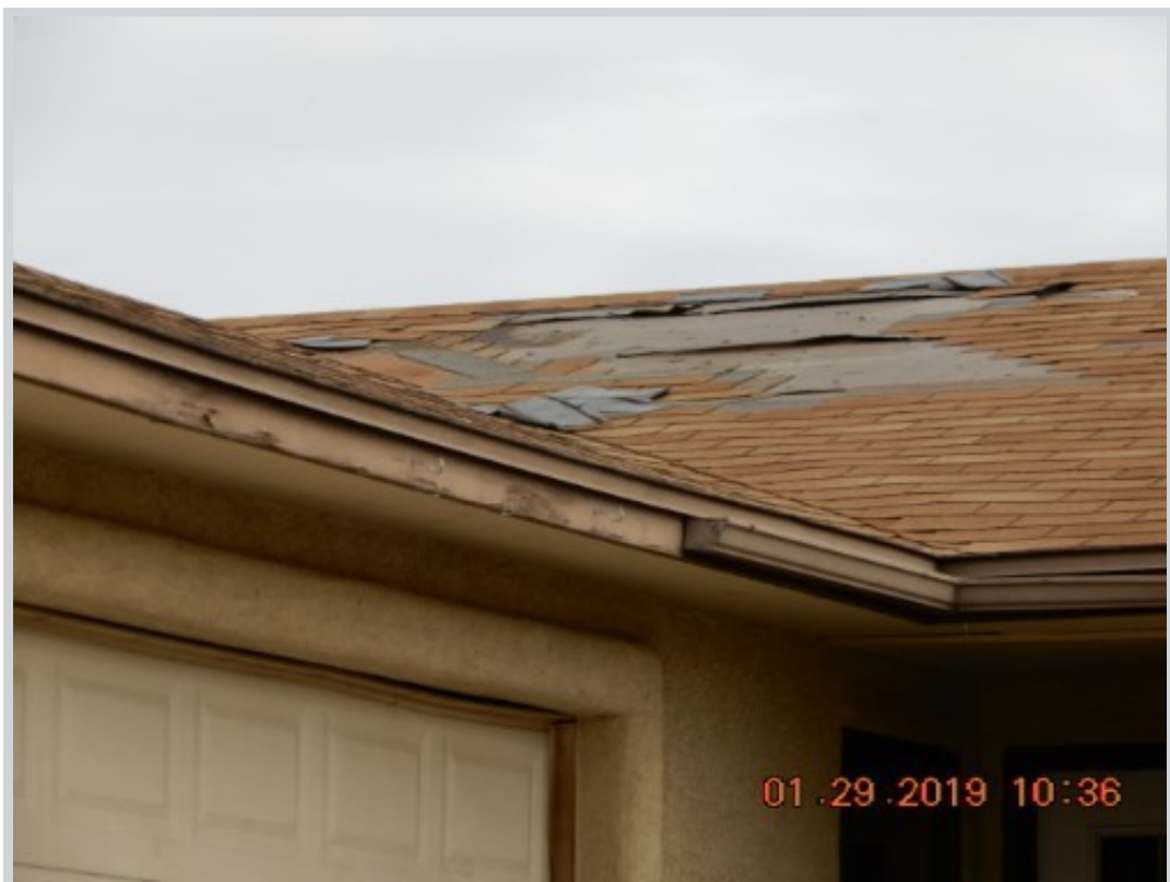
Subject 221 Veeder Dr View Other Comment "Area of damaged composition shingles. "
