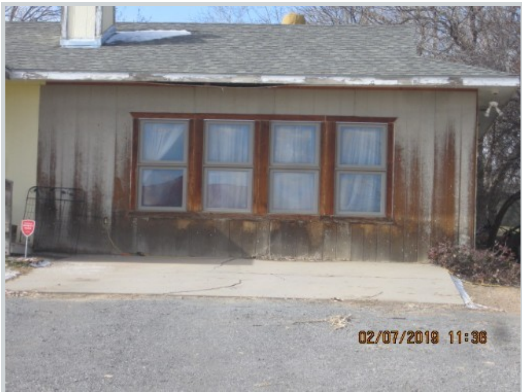
Subject 1329 Dublin Drive Dr View Other Comment "paint damage"
