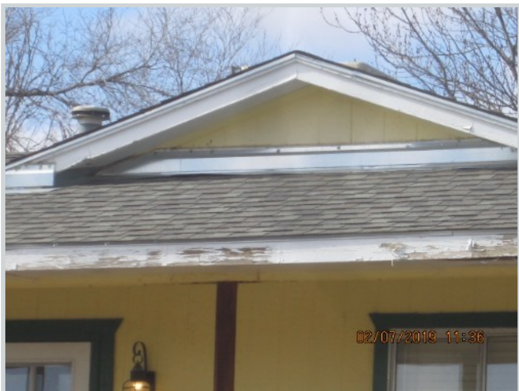
Subject 1329 Dublin Drive Dr View Other Comment "trim paint damage"
