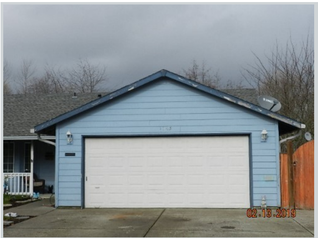
Subject 1345 33rd Pl View Other Comment "damage paint trim"
