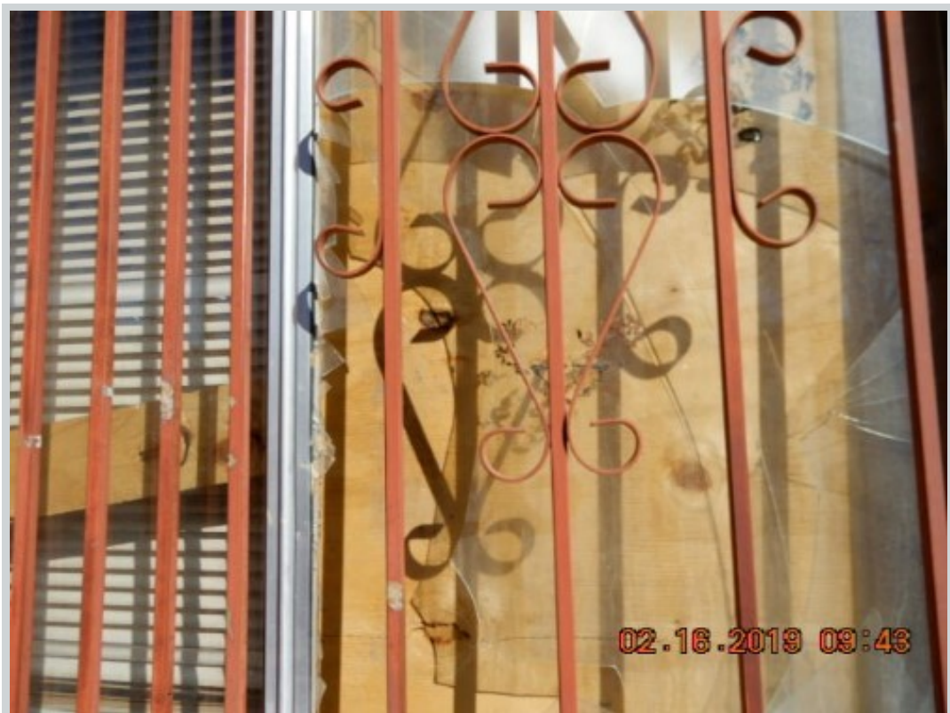
Subject 2117 Cameron St View Other Comment "Cracked window. "
