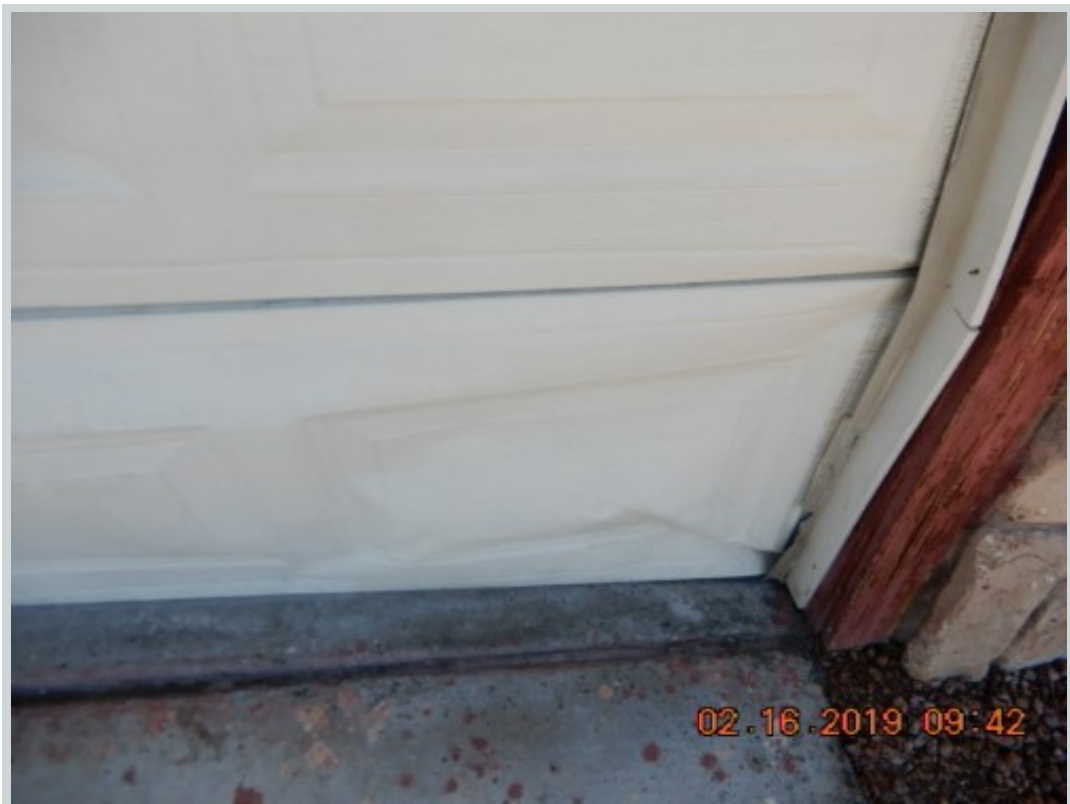
Subject 2117 Cameron St View Other Comment "Garage door is damaged. "
