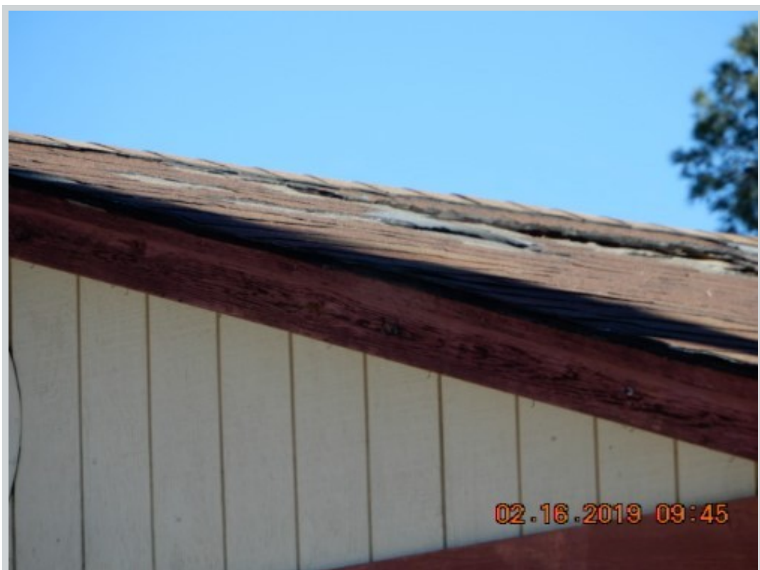
Subject 2117 Cameron St Comment "Small area of damaged composition shingles. "
