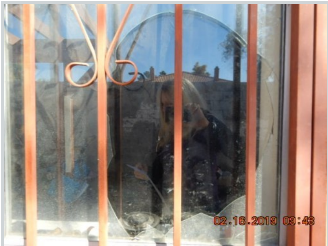
Subject 2117 Cameron St Comment "Cracked window. "
