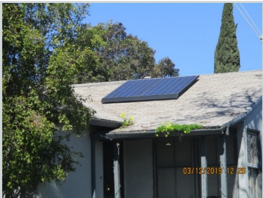
Subject 1112 W 8th St View Other Comment "Solar panels on roof, unknown if owned or leased. Also, gutters need to be cleaned."
