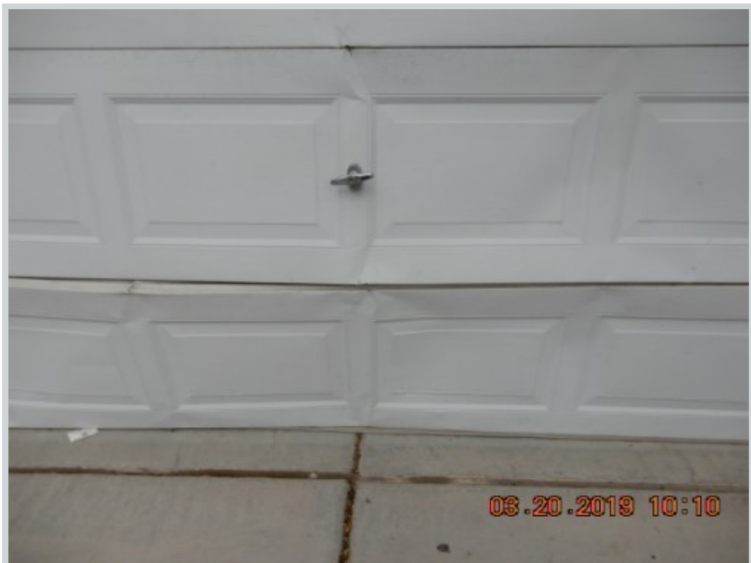
Subject 4186 Dobson Dr View Other Comment "Damaged garage door. "
