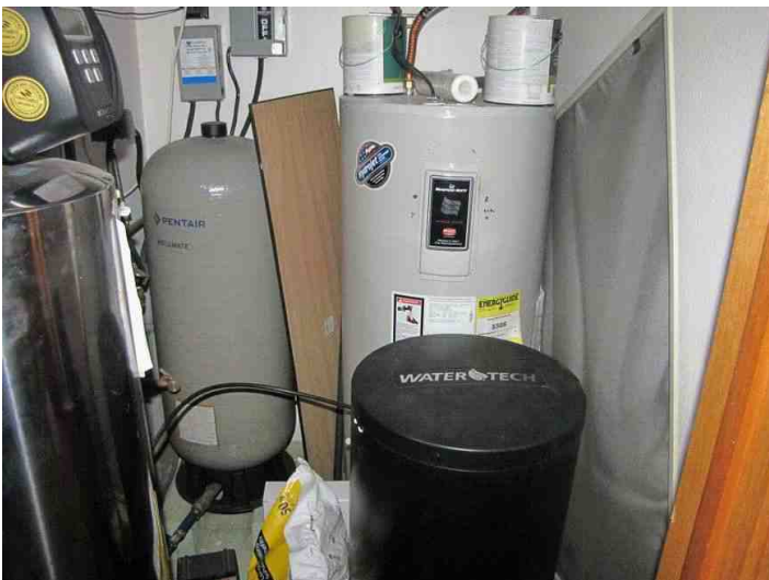
Hot Water Tank
