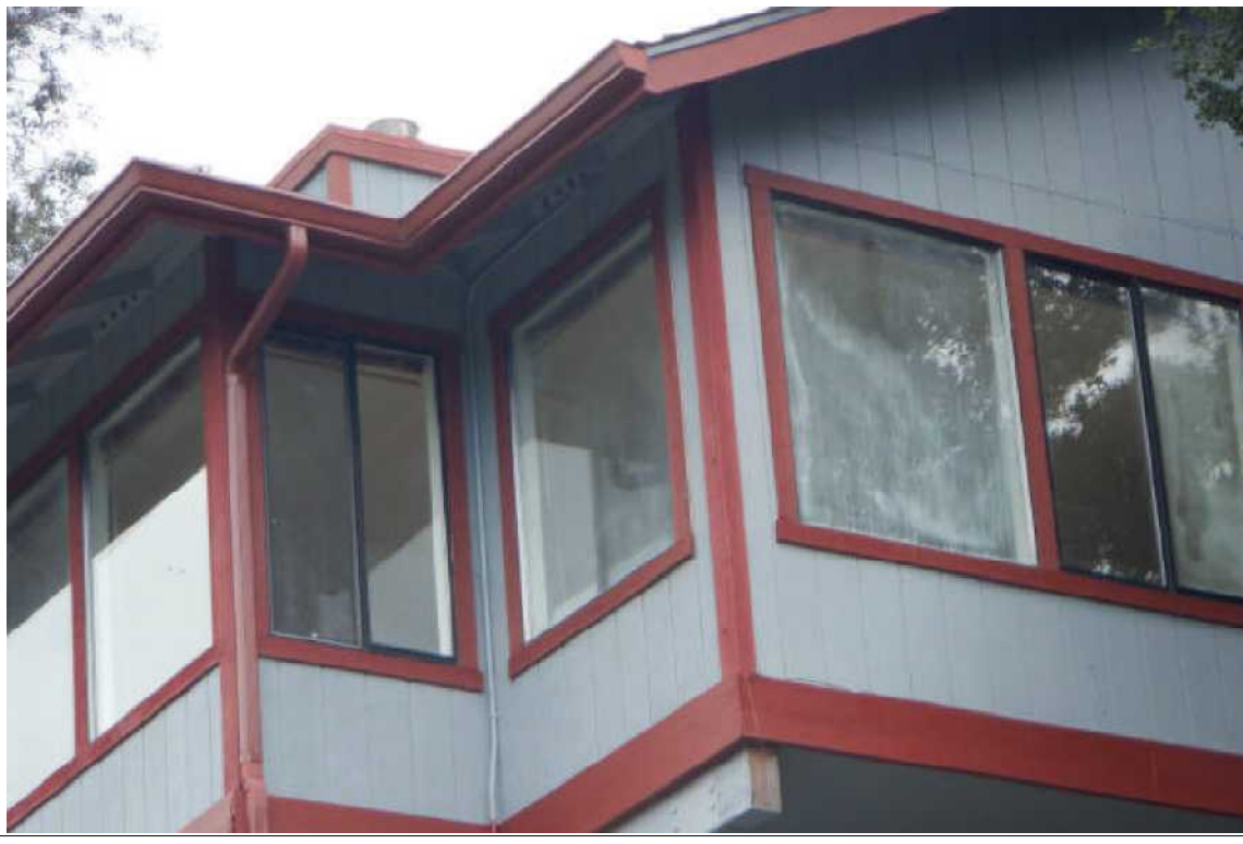
Windows appear to have lost seal
