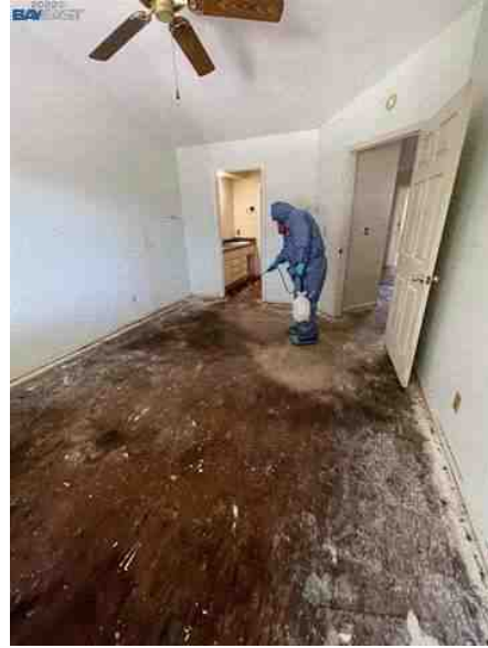
MLS PHOTO: Worker appears to be treating mold
