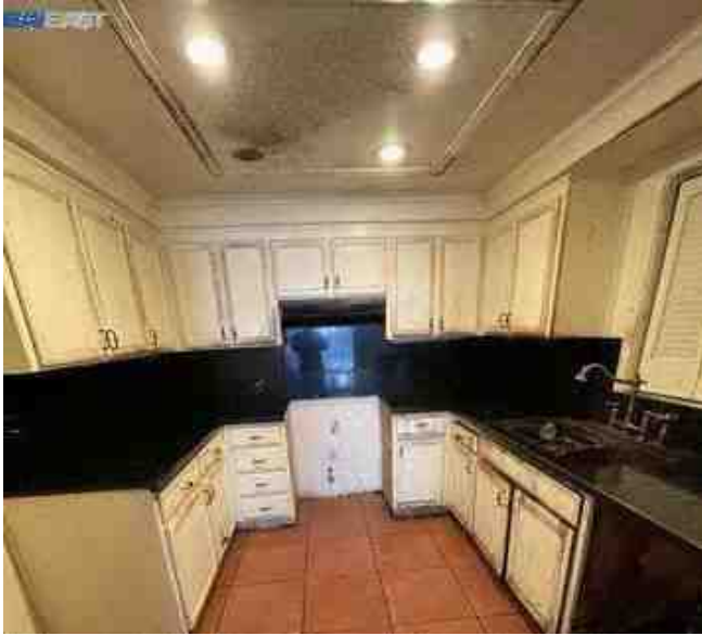
MLS PHOTO: Appears to be mold on ceiling and cabinets
