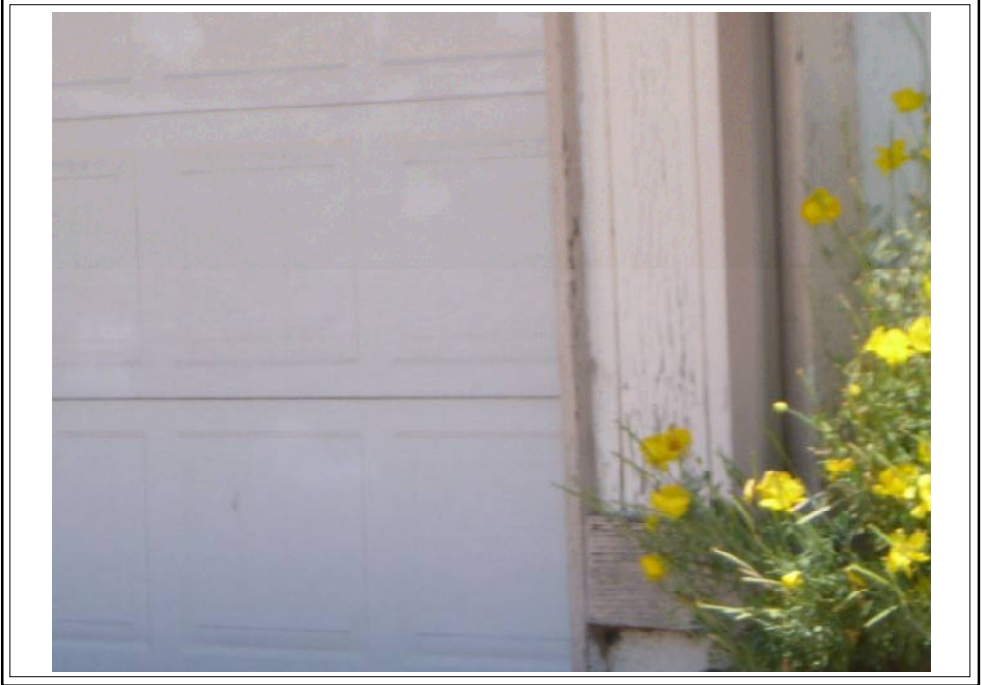
Deferred Maintenance (peeling paint)
