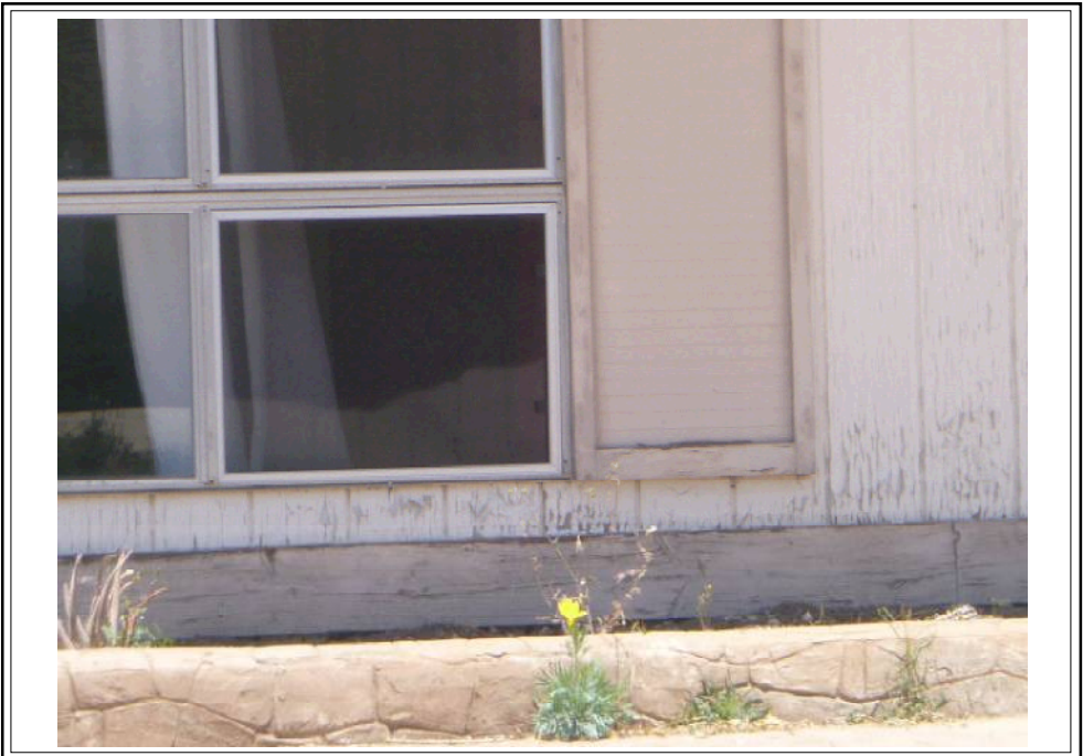
Deferred Maintenance (peeling paint)
