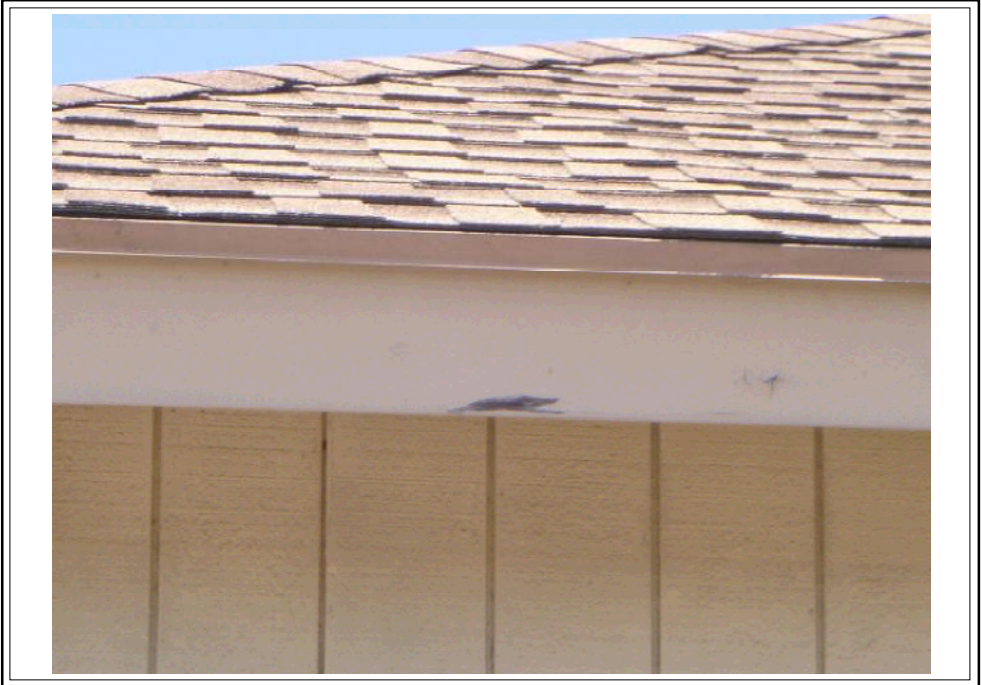
Deferred Maintenance (peeling paint)
