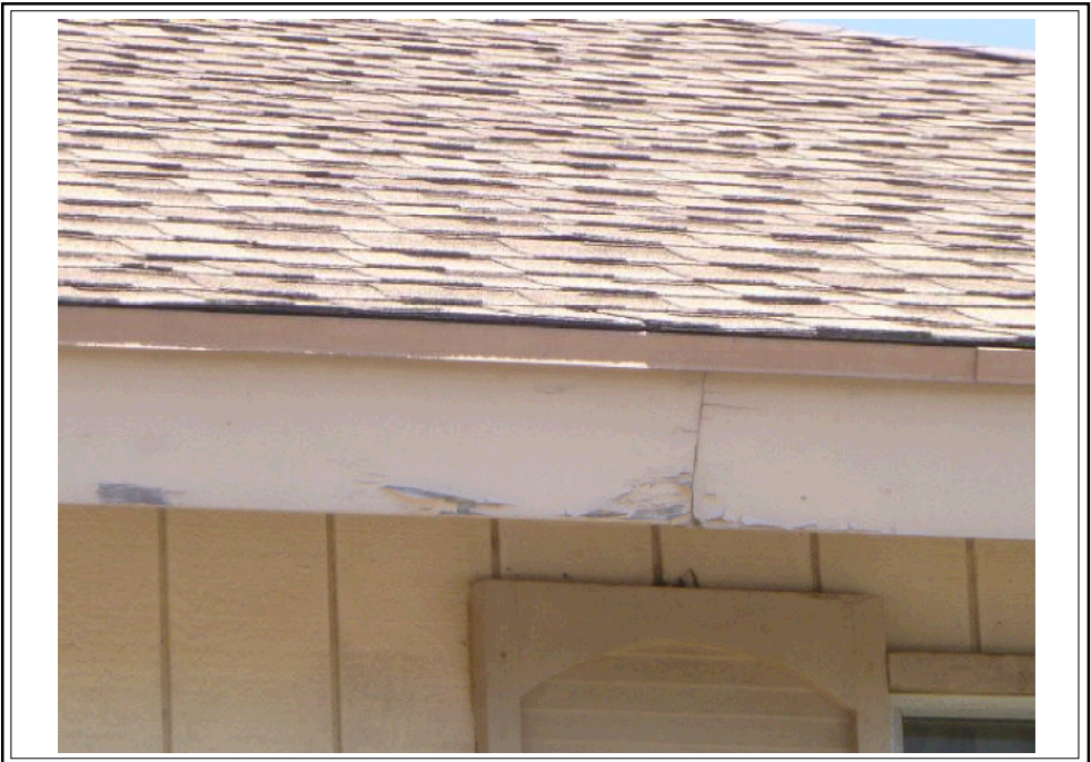
Deferred Maintenance (peeling paint)
