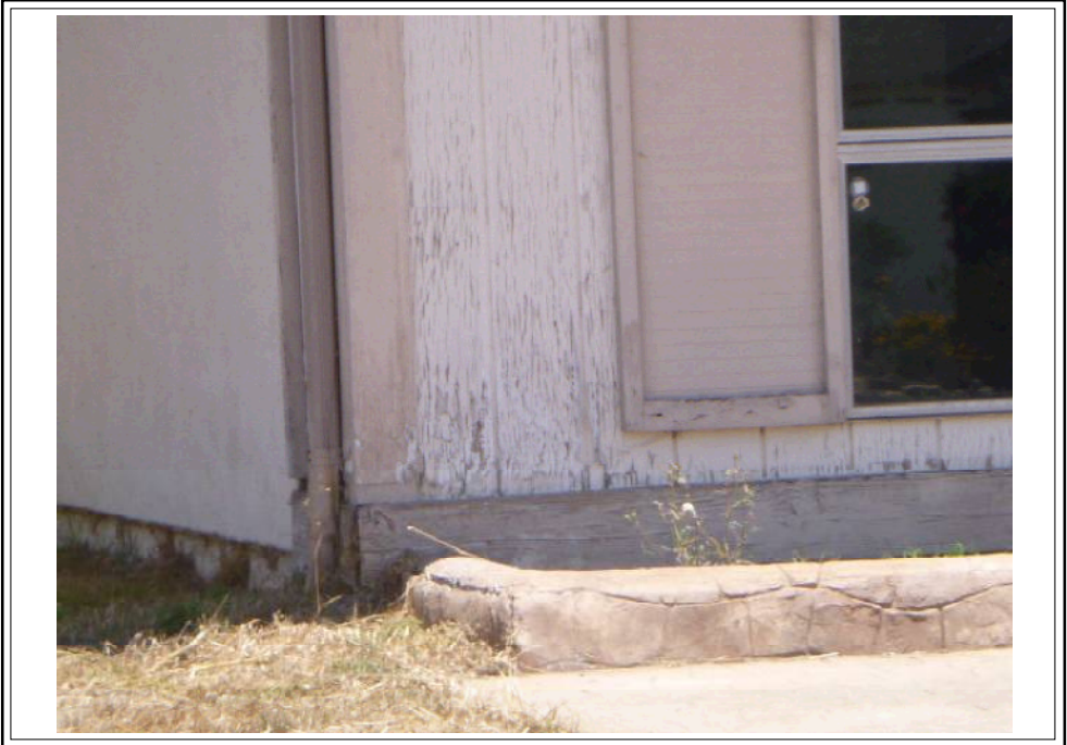
Deferred Maintenance (peeling paint)
