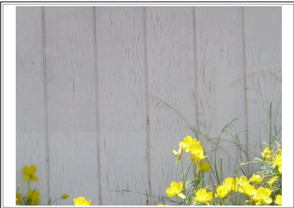
Deferred Maintenance (peeling paint)
