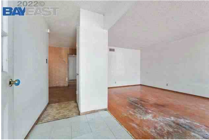
Discoloration on Wood Flooring
