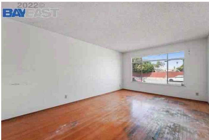
Discoloration on Wood Flooring
