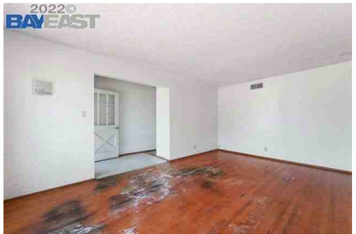
Discoloration on Wood Flooring
