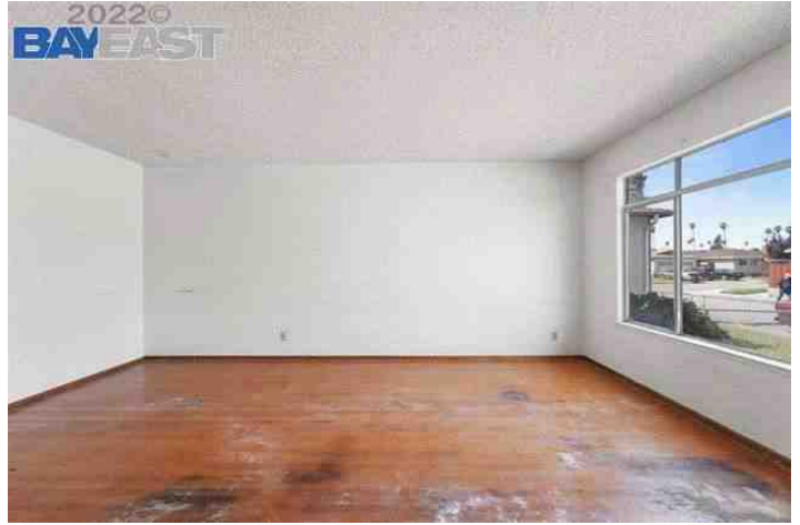
Discoloration on Wood Flooring
