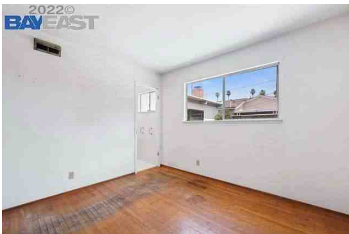
Discoloration on Wood Flooring
