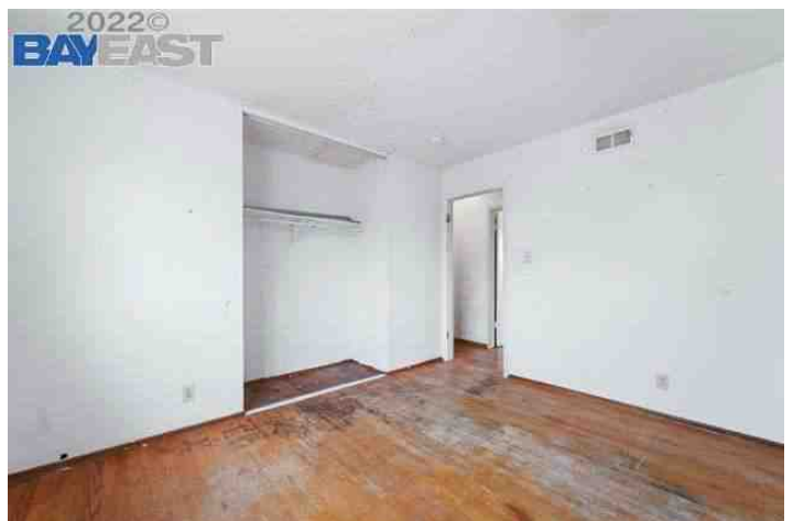
Discoloration on Wood Flooring
