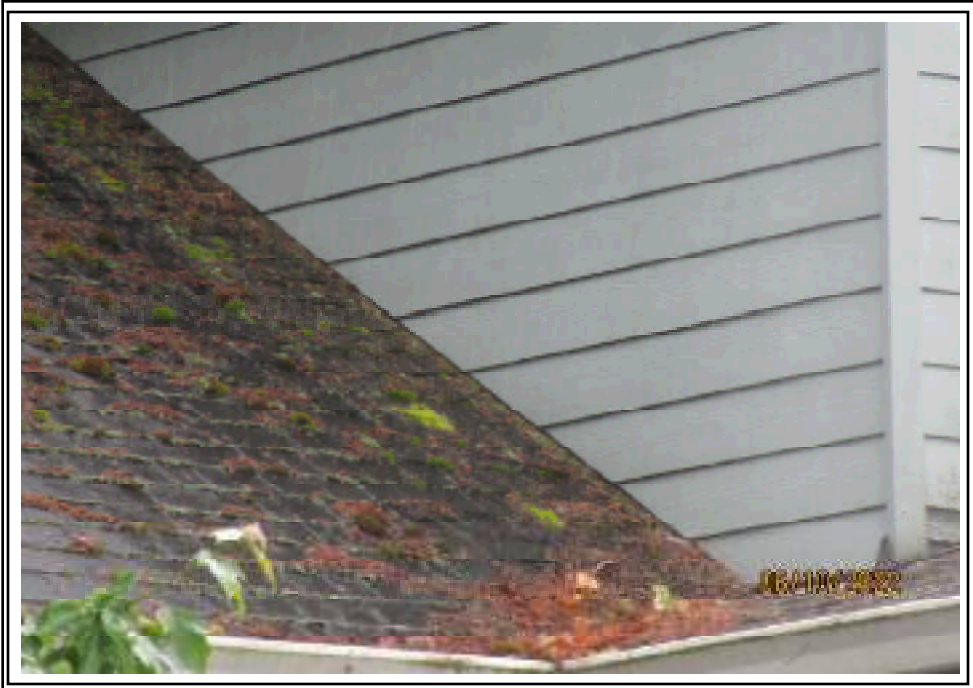
Moss noted on the roof cover
