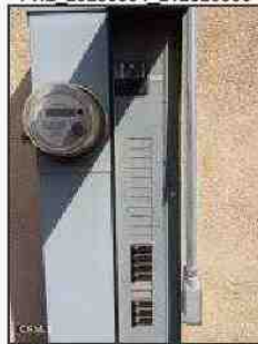
Newer electrical panel
