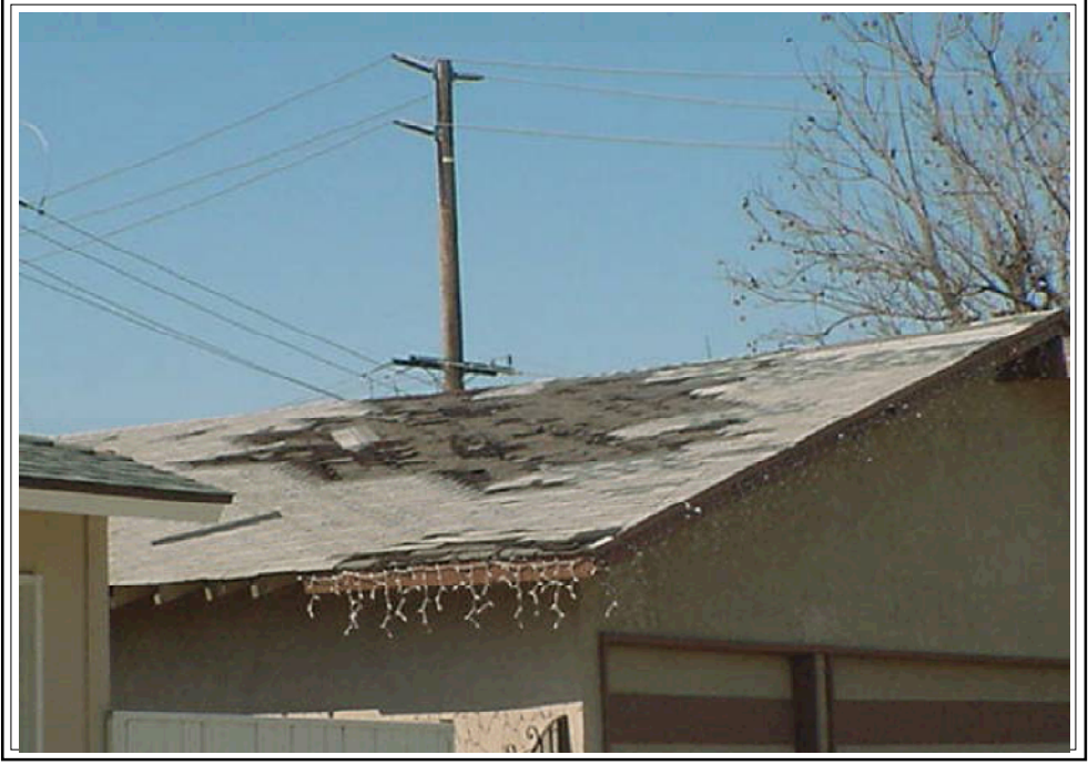
WORN ROOFING OVER GARAGE
