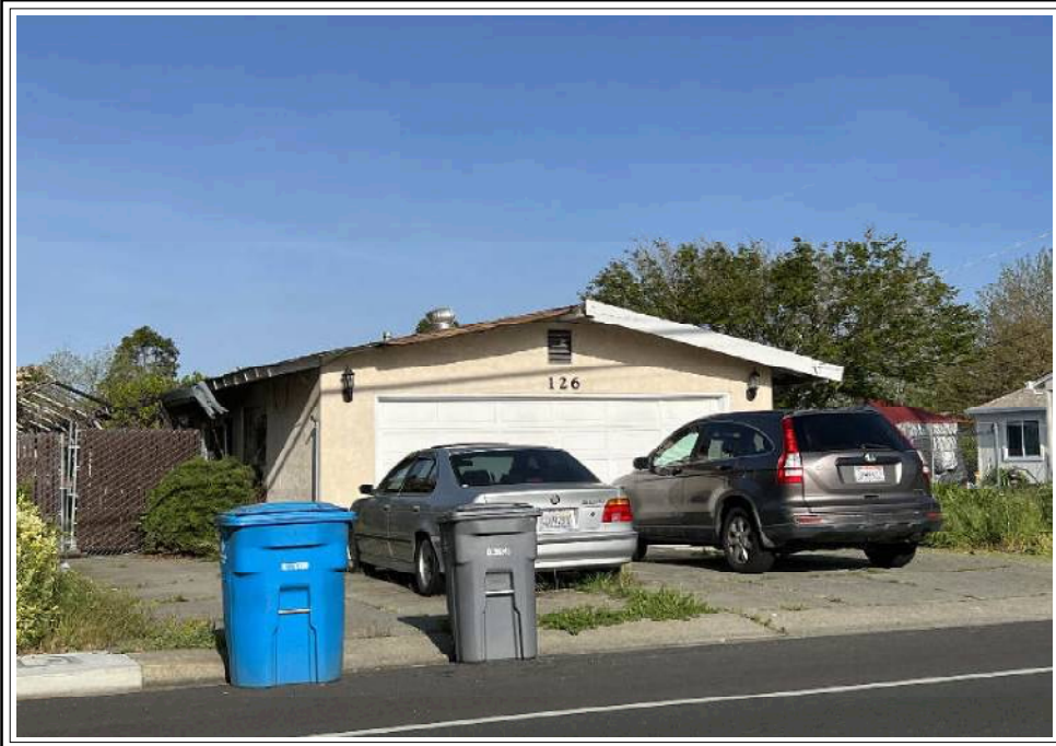
ADDRESS FRONT FASCIA MISSING
