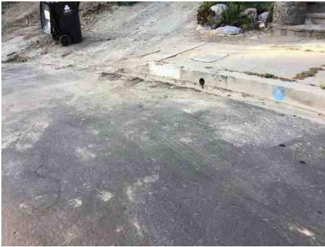
Curb address washed away
