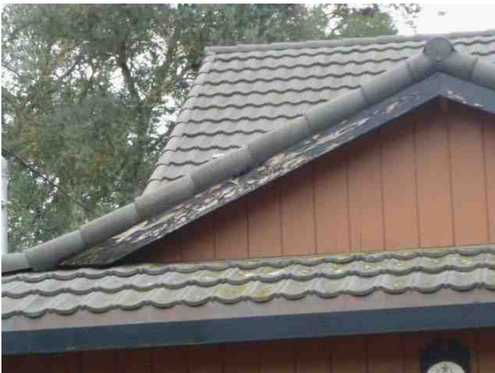
Cracked and peeling paint on trim
