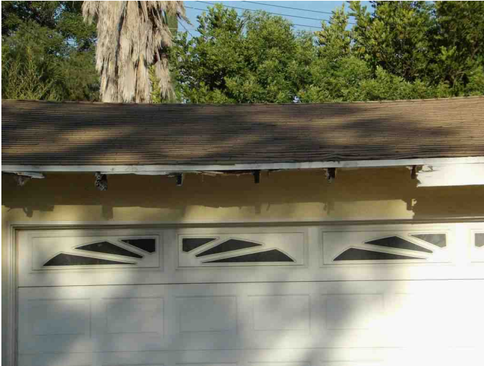
WOOD TRIM DRY ROT
