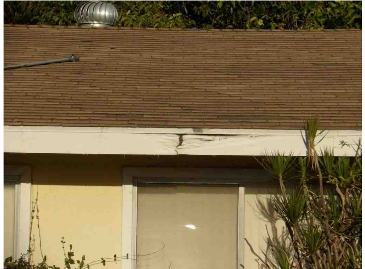
WOOD TRIM DRY ROT
